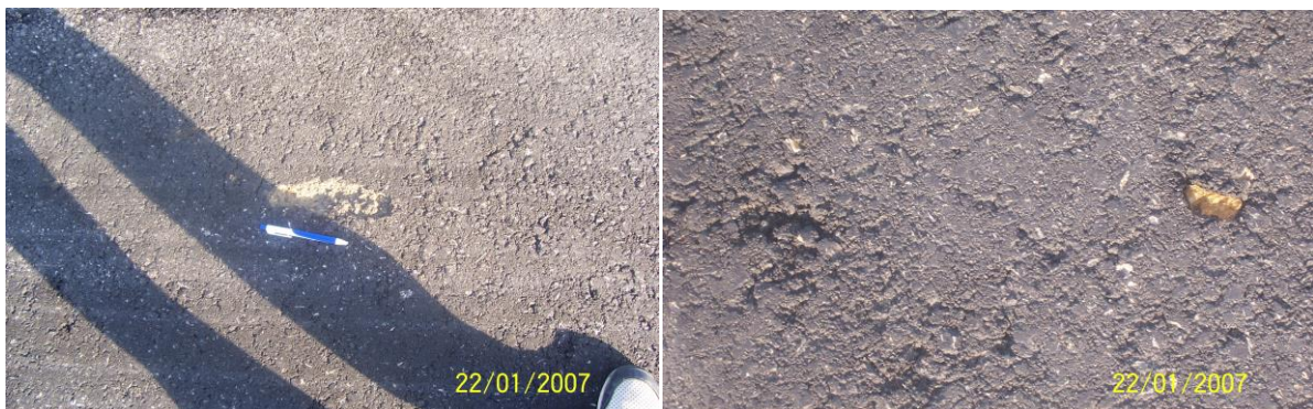
Picture 1. Distressed Asphalt (Source: Pictures taken from the construction site)
